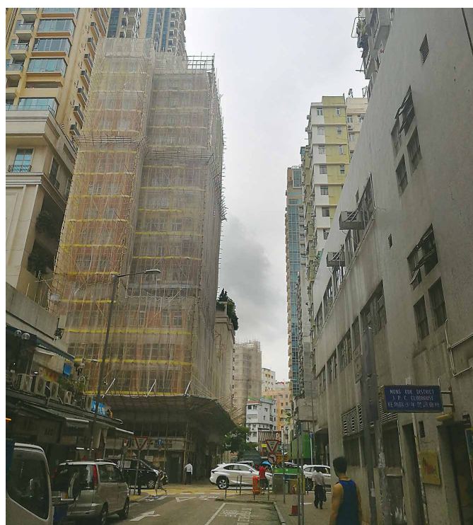
Figure 6: Double-row bamboo scaffold for building maintenance works
